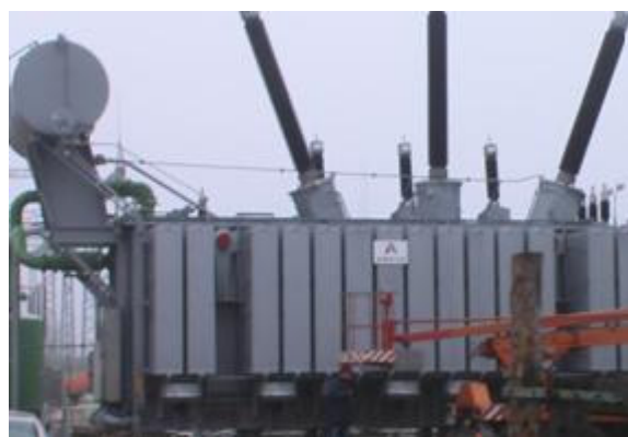
Fig.1 The autotransformer 400/121/34 kV
