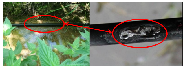
Fig. 1: The consequence of failure - Conductor fallen on the ground.
