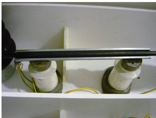
Fig. 4: Example of fault simulation in laboratory conditions: Analysis of CC discharge activity in fault condition at temperature of 20 \text{ }^\circ\text{C} . Drop of conductor onto pole console.
