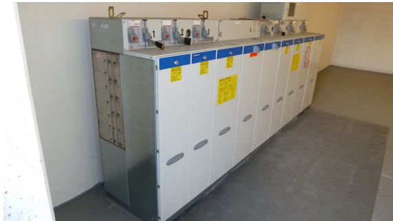
Fig. 2: MW switchboard of the customer Magna (node U3 according to Fig. 1).
